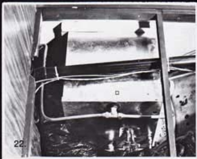
THE 6.2 GALLON FAST RECOVERY HEAT EXCHANGER HOT WATER HEATER □ IS LOCATED FOR EASY ACCESS IN THE KITCHEN AREA. NO MORE WAITING FOR THE HOT WATER.
